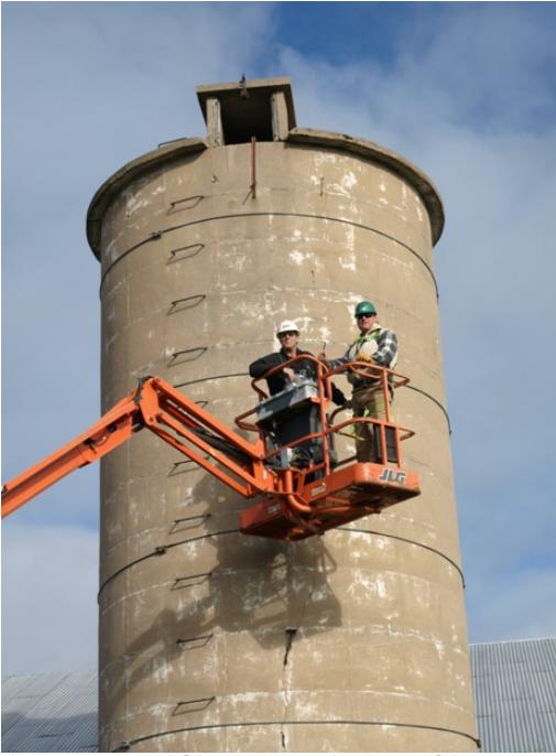
Figure 7: Monolithic concrete silo located in Oconto County, Wisconsin built in 1919. Note the dormer window and the attached ladder. This silo also features reinforcing hoops and due to the weathering of the paint, the slip form seams are now visible.
