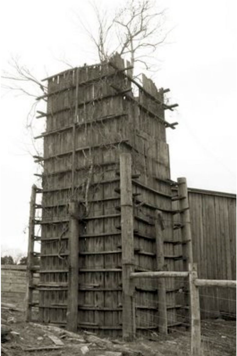
Figure 1: Rectangular silo built on the exterior of a barn. Note the substantial efforts at additional structural support and bracing to hold back the pressures of the silage. Location unknown.
