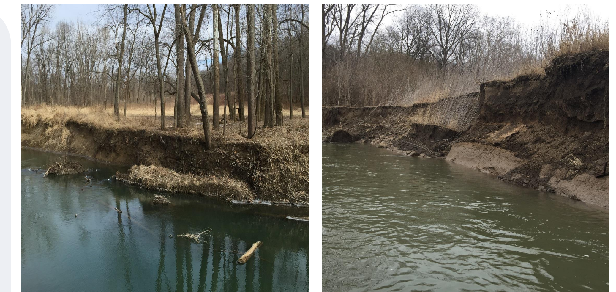
Figure 6 (left). Bank failure at the upstream corner of the entrance to the chute cutoff. Figure 7 (right). Bank erosion along the cut bank at the downstream end of the main channel.
